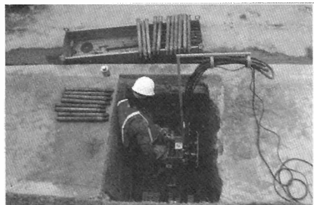
FIGURE 24 Pit launched mini-horizontal directional drilling (63): (Top) The block wall eliminated options for drilling without damage to curb or street. (Bottom) The quick shot requires a compact setup pit. With this model, only a 3-ft by 4-ft pit, half of a sidewalk flag, at this site.
