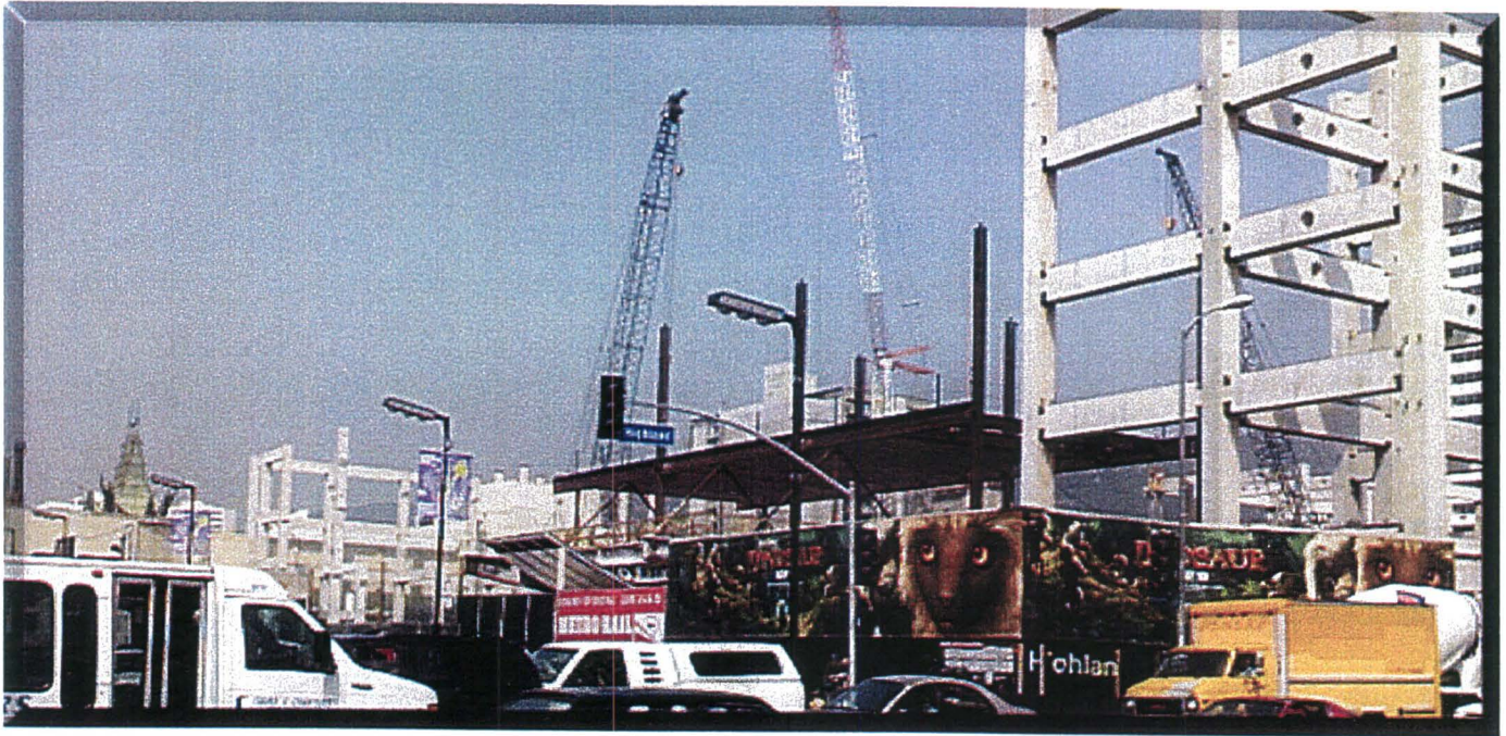
K5: View is facing the northwest corner of Hollywood Boulevard and Highland Avenue, the future home of the Redline Hollywood & Highland Metro Station and mixed use commercial project (i.e., The “Hollywood & Highland” project site).
