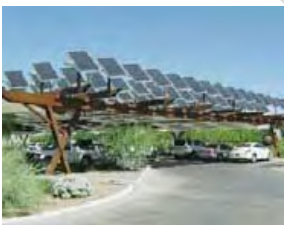
Solar panel shade structure
