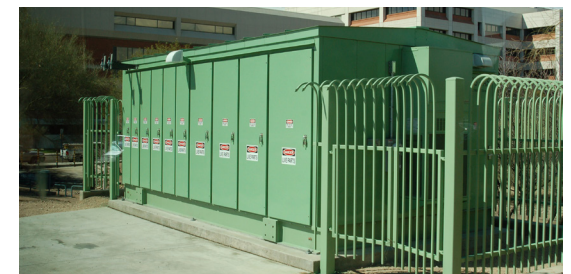
Source: AECOM Figure 2.8-2 Example Traction Power Substation
