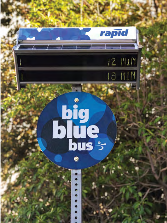
Arrival time displays give riders valuable information. Some models, such as this one, are solar-powered. Photo courtesy of Big Blue Bus.
