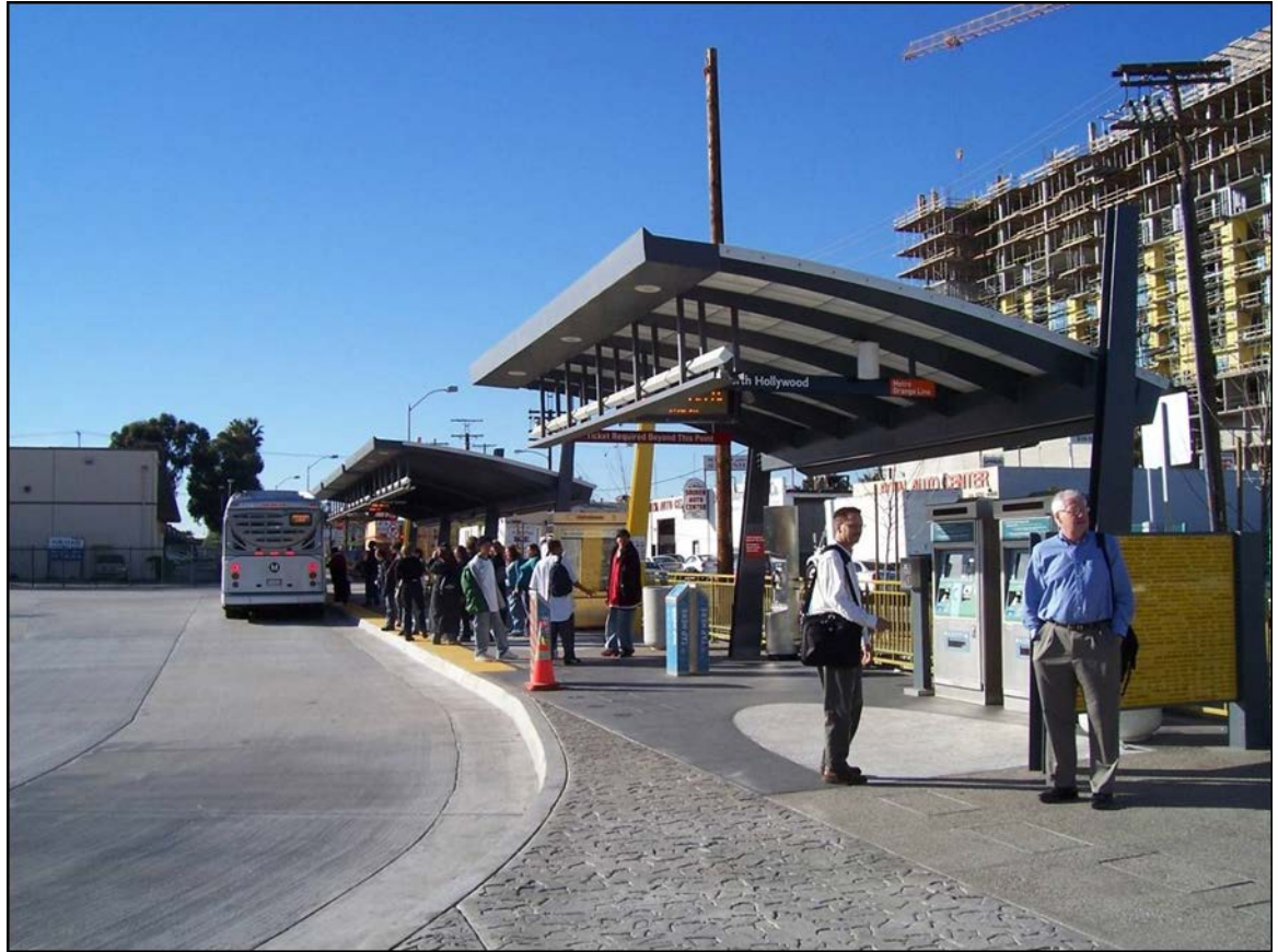
Figure 5-4 Construction at Orange Line Terminus and Red Line Connection at North Hollywood Station
