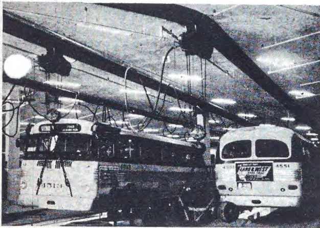
Heavy lifting is performed by air-controlled hoists and mono-rail cranes.
