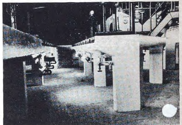
This close up shows the open pit construction being employed in the new DSR garages.
