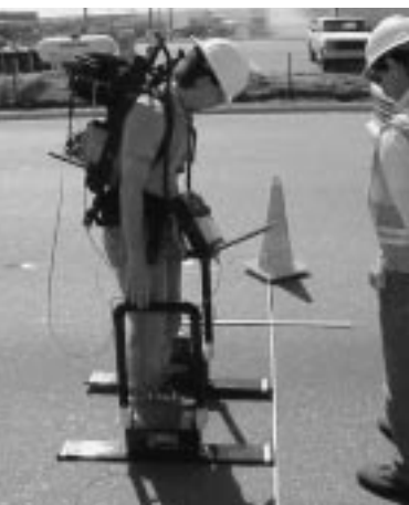
Practitioners need more non-destructive testing methods, like ground-penetrating radar, used to locate subsurface obstructions.
