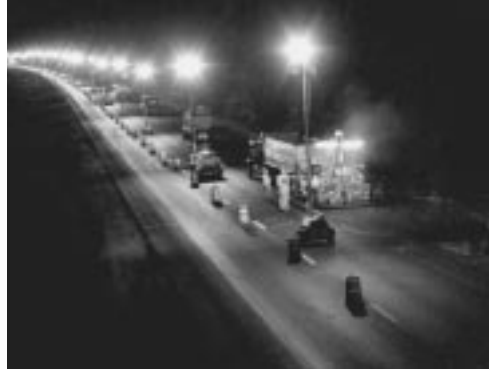
Nighttime construction and maintenance, subjects of NCHRP Reports 475 and 476, are now common on heavily traveled roads.
