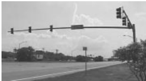
Traffic signal mast-arm of the type detailed in NCHRP Report 469, Fatigue-Resistant Design of Cantilevered Signal, Sign, and Light Supports .
