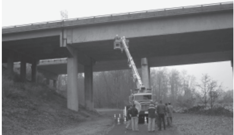
Members of the Committee for Review of the Oregon Department of Transportation Study on Bridge Shear traveled to Oregon to conduct a site inspection of bridges with cracked girders, as part of a peer review of an Oregon State University study.
