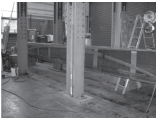
Hillman composite bridge beam is prepared for testing under a project funded by NCHRP IDEA and High-Speed Rail IDEA.
