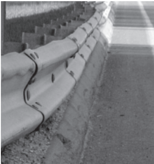
Recommended guidelines for curb and barrier installations are presented in NCHRP Report 537.
