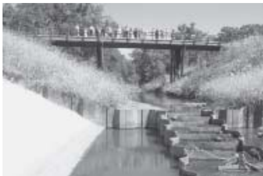
Sheet pile weir fitted with a fish ladder, to prevent streambed degradation and enable fish to migrate upstream, from NCHRP Report 587, Countermeasures to Protect Bridge Abutments from Scour .
