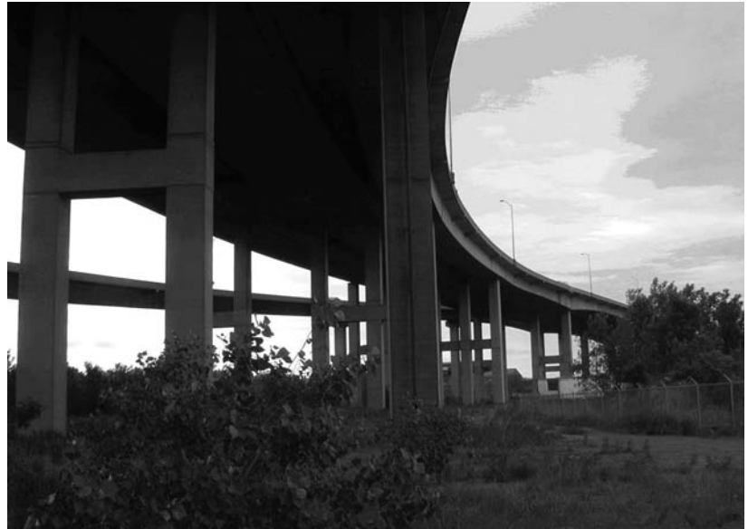
A cast-in-place box girder bridge was a case study for the nondestructive evaluation of corrosion, discussed in a paper included in web Circular E-C 128, 10th International Conference on Bridge and Structure Management . 5
