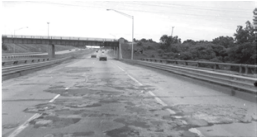
Repairs of critical roughness on a concrete bridge deck, from Transportation Research Circular E-C134, Influence of Roadway Surface Discontinuities on Safety: State of the Art Report .
