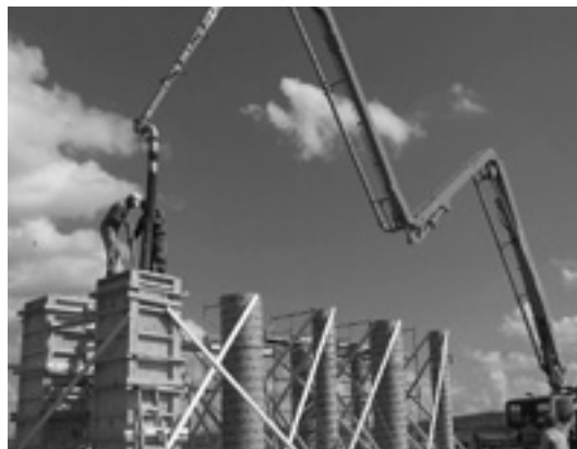
Half-scale reinforced concrete bridge columns for Phase II testing described in NCHRP Report 645 are cast with a concrete pump truck and consolidated with a hand vibrator at the Southwest Research Institute test site in Yancey, Texas.
