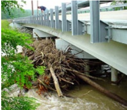
NCHRP Report 653 examines the effects of debris on bridge scour. At this bridge, a fully formed mass of debris creates significant scour potential.
