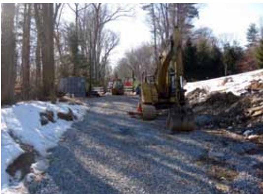
Gaining federal aid for small-scale local projects, such as this road widening in Radnor Township, Pennsylvania, is the subject of NCHRP Synthesis 414. (Photo: Leslie McCarthy)
