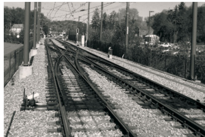
TCRP Report 155 explores the design of common light rail transit track types.
