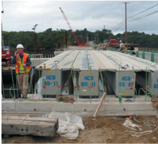
Hybrid composite beams—developed with support from the NCHRP IDEA program—are used in the construction of the Knickerbocker Bridge in Boothbay, Maine. (Photo courtesy Dale Peabody, Maine DOT)
