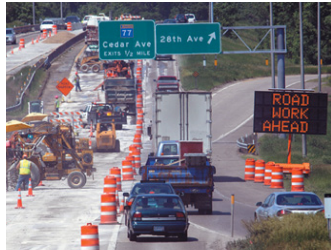
Annual Meeting sessions hosted by the Maintenance and Preservation Section committees examined work zone safety and mobility, driver behavior in work zones, and other topics. (Photo: Minnesota DOT)
