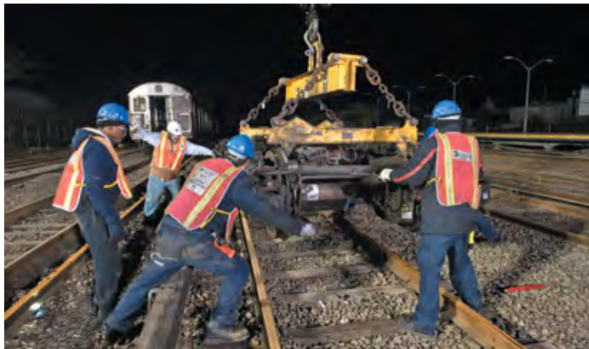
New York City transit crew works to restore service after storm flooding. Superstorm Sandy was the topic of a special Annual Meeting session sponsored by the Critical Transportation Infrastructure Protection Committee and the Task Force on Disaster Response and Business Continuity. (Photo: Metropolitan Transportation Authority)
