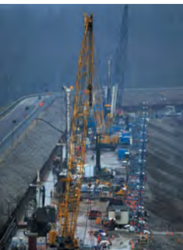
The U.S. Army Corps of Engineers Nashville District oversees a foundation remediation project to stop seepage at the Wolf Creek Dam in Jamestown, Kentucky. The needs of the U.S. Inland Waterway System are the subject of a current TRB policy study. (Photo: Leon Roberts, USACE)
