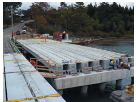
The award-winning hybrid composite bridge beam, used in the construction of Knickerbocker Bridge in Boothbay, Maine, was developed with assistance from the Innovations Deserving Exploratory Analysis program.
