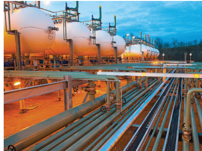
A liquid natural gas production plant in Ohio. Natural gas pipelines are the subject of HMCRP Report 14, Guide for Communicating Emergency Response Information for Natural Gas and Hazardous Liquid Pipelines . (Photo: Bilfinger SE)
