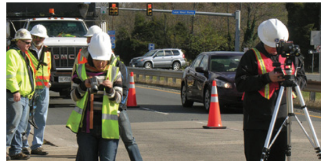
Nondestructive testing products developed as part of SHRP 2 Renewal research are in use across the United States. (Photo: Nenad Gucunski, Rutgers University)
