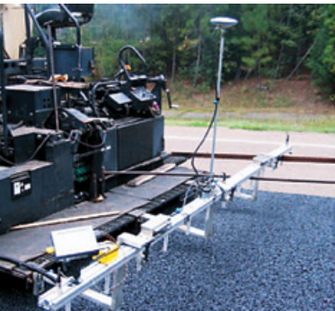
Nondestructive technologies such as Pave-IR for detecting defects in asphalt pavements during construction were pilot tested in Vermont in conjunction with FHWA's Every Day Counts program.
