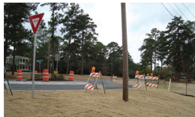
A new roundabout under construction in Valdosta, Georgia. The Safety and Systems Users Group sponsored a popular series of webinars on roundabouts, addressing such topics as accessibility, advances in roundabout design, and trucks and oversized loads. (Photo: Valdosta-Lowndes Metropolitan Planning Organization)
