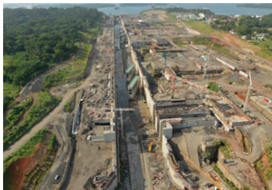
Construction on the Atlantic Lock, part of the Panama Canal expansion program. In commemoration of the centennial of the canal, the Freight Systems Group sponsored an Annual Meeting workshop focused on the history and future of the canal. (Photo: Courtesy of the Panama Canal Authority)
