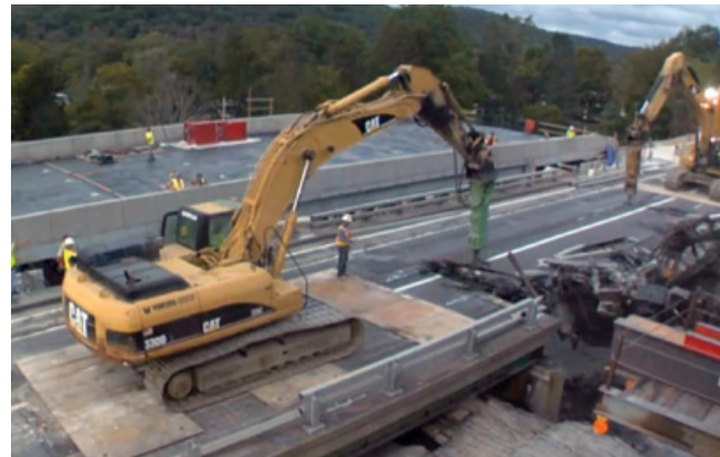
Video still from a weekend replacement of two bridge spans using accelerated bridge construction technology. The new bridge was built on site, then the old bridge was demolished and the new one slid into place.
