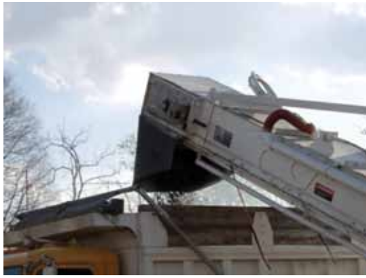
Hot-mix asphalt delivered from a material transfer vehicle, an example of the techniques presented in Transportation Research E-Circular 198, Moisture Damage to Hot-Mix Asphalt Mixtures .
