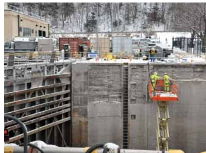
Maintenance on Lock and Dam 8 near Genoa, Wisconsin. The U.S. inland waterways system was the subject of a TRB policy study. (Photo: Patrick Moes, U.S. Army Corps of Engineers)
