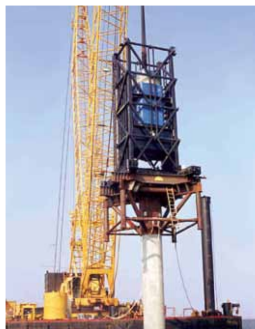
Statnamic load tests at St. George Island Bridge, as addressed in NCHRP Synthesis 478, Design and Load Testing of Large-Diameter, Open-Ended Driven Piles . (Photo copyright Applied Foundation Testing)
