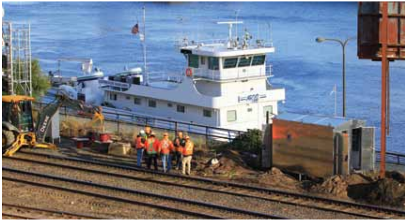
Railroad workers handle signal cables in the Saint Paul Union Depot in Minnesota. Workforce capacity is an area of focus in the National Cooperative Rail Research Program. (Photo: Michael Hicks)
