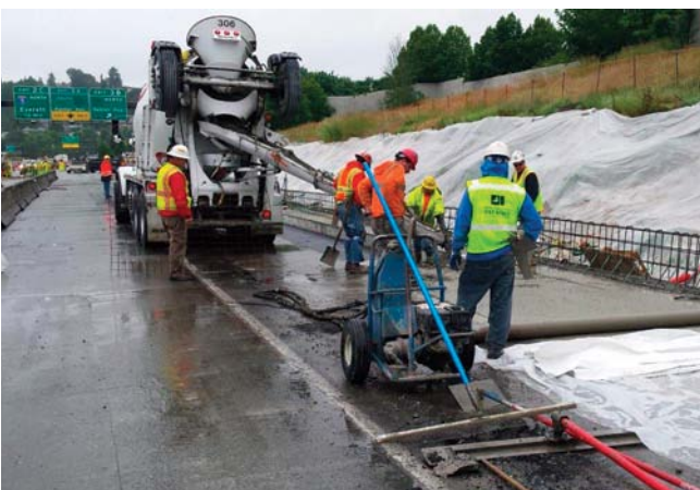
Crews place new concrete pavement on westbound I-90 in Washington State. Concrete and Asphalt Materials Sections activities examined durable concrete, long-life concrete, concrete quality sensors, and more. (Photo: Washington State DOT)
