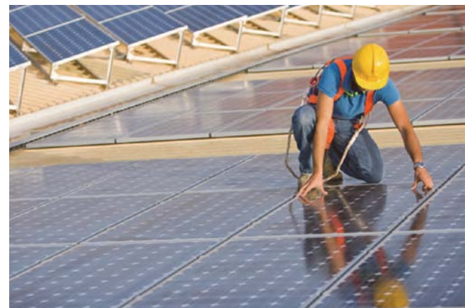
Installation of solar panels at an airport facility, from ACRP Report 151, Developing a Business Case for Renewable Energy at Airports .
