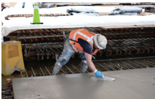
Construction of an interior precast panel for one of the SR-520 bridge pontoons in Washington State. Committees in the Construction and Materials Sections organized workshops on such topics as precast concrete pavement technologies. (Photo: Washington State DOT)
