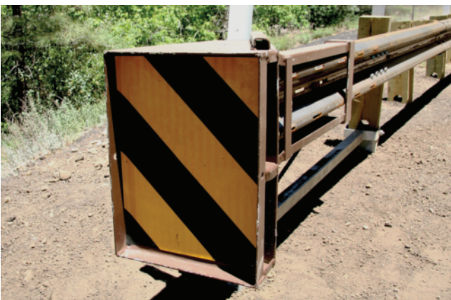
Special Report 323, In-Service Performance Evaluation of Guardrail End Treatments , offers guidance for highway agencies in selecting, maintaining, and replacing guardrail end treatments. (Photo: Arizona DOT)
