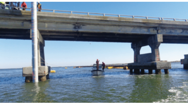
Test piles driven before a bridge replacement in coastal North Carolina. Environment and Energy Section committees examined noise and vibration impacts and other environment-related topics at their conferences in 2017. (Photo: North Carolina DOT)
