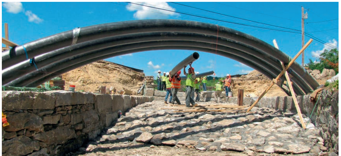
Massachusetts deployed bridge-in-a-backpack materials in a Fitchburg bridge replacement. Bridge-in-a-backpack technology was among those funded by a federal innovative bridge research program. (Photo: Massachusetts Department of Transportation)
