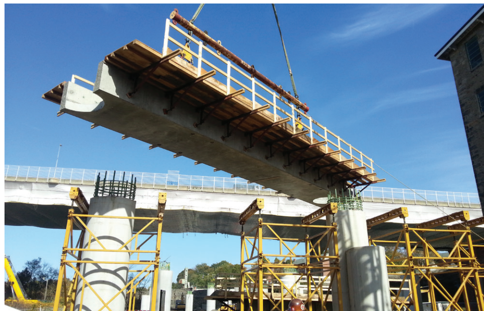
Massachusetts DOT lifts a precast bridge deck into place. Special Report 330 examines the success of innovative techniques like accelerated bridge construction. (Photo: Massachusetts DOT)
