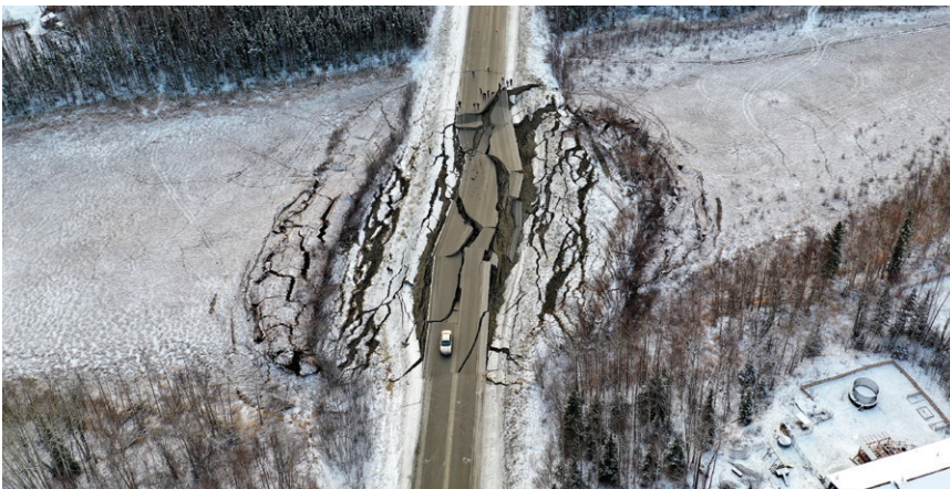
A series of earthquakes in Alaska destroyed highway infrastructure in 2018. New TRB subcommittees examine systems resilience and managing supply chain disruptions during and after natural disasters. (Photo: Alaska DOT)
