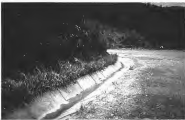
FIGURE 10 Vetiver used to protect edge of road drain from sedimentation and small rock fill in Doi Tun, Thailand. Note clean drain, which saves annual maintenance costs and ensures that drain functions when needed (photograph by R. G. Grimshaw).
