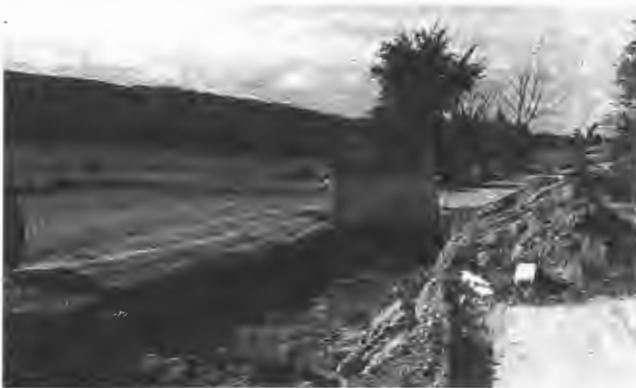
FIGURE 6 Roadway excavation included stockpiling of \pm 22 in. of existing gravel and disposal of 8 to 12 in. of silty sand subgrade.
