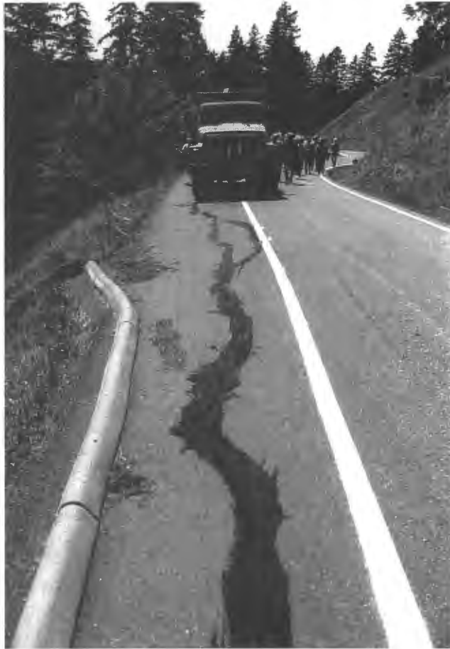
FIGURE 8 Failing road shoulder typical of those needing stabilization.
