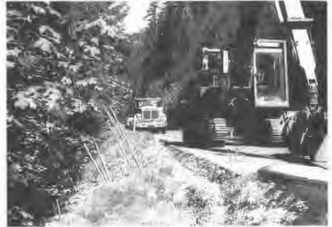
FIGURE 5 Nails installed in road shoulder without disturbing vegetation. Nails were cut off at ground surface. Note pavement displacement in right foreground (1).
