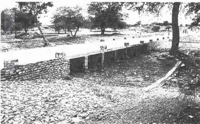
FIGURE 3 Stone masonry bridge (note guide blocks on deck and gabions and cut-off wall in foreground).
