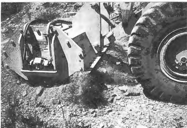
FIGURE 7 Roto Trimmer in operation; note small amount of dust and sidecast material.
