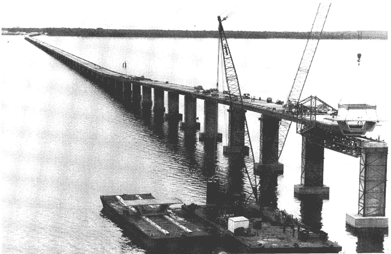
FIGURE 3 Typical 41.5-m (135-ft) spans were erected by span-by-span methods by using an assembly truss. The contractor was routinely able to erect four spans per week. During the week of September 20, 1992, the contractor was able to erect seven spans in 7 days [290 m (952 ft) of completed bridge in 1 week], a world record for span-by-span erection speed.
