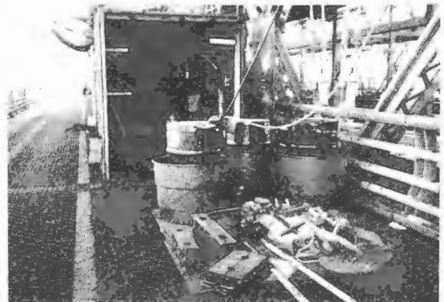
FIGURE 4 Containment system for main cable oiling: top , troughs for dripping oil; bottom , oil conveyed by hoses to disposal drums.
