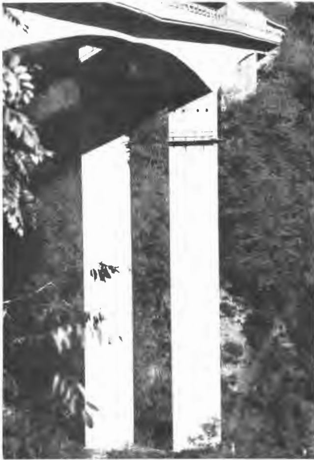
FIGURE 8 Ruiz Viaduct before repair. A large deflection at midspan is visible to the naked eye.
