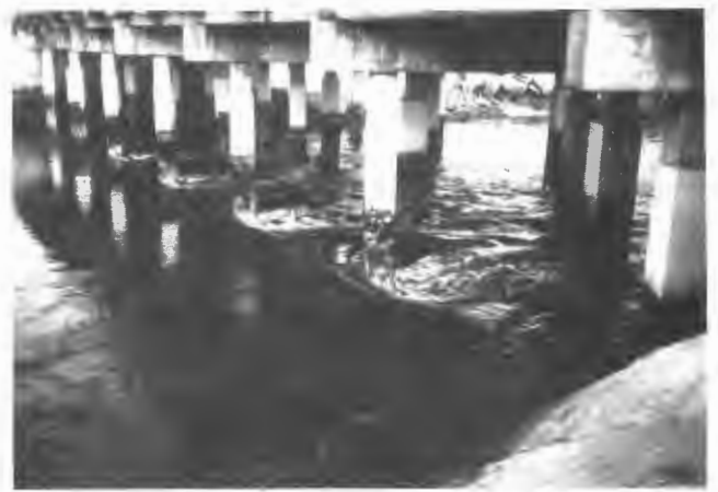
FIGURE 5 Bridge over Shad Creek, just above confluence with St. John's River, Jacksonville, District 2, FDOT.
