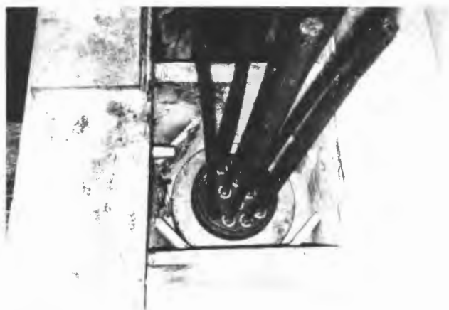
FIGURE 12 Steel frame placed at end of each beam to anchor new cables.
