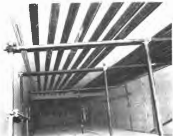
FIGURE 10 External cables added inside Stupino Viaduct. HDPE sheets were grouted with cement-mortar.
