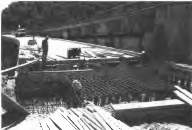
FIGURE 2 New abutment built to withstand longitudinal horizontal forces; in front, deck with continuous slab.
