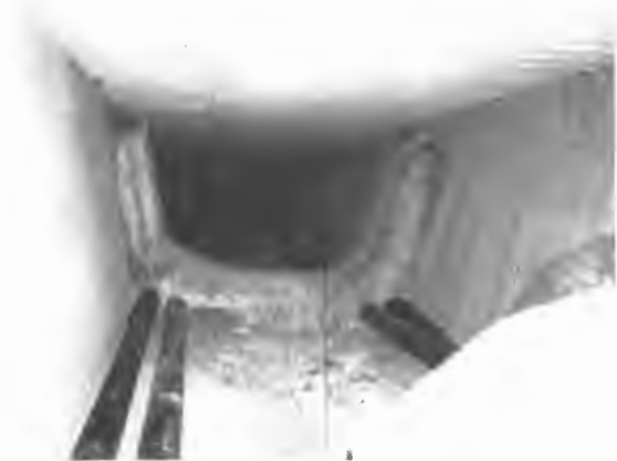
FIGURE 11 Deviation block added inside box girder. The external prestressing cables are composed of single sheeted strands. They will not be grouted.
