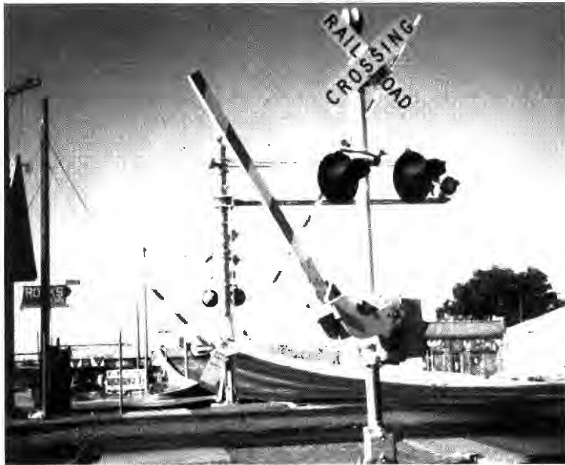
FIGURE 7 Pedestrian automatic gate examples: top , Option A, Skokie, Illinois; bottom , Option B, Holbrook, Arizona.
