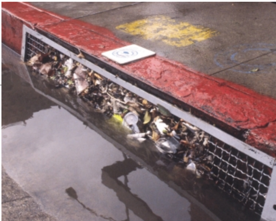
A Santa Monica storm drain opening captures street litter, preventing trash from reaching the ocean.
