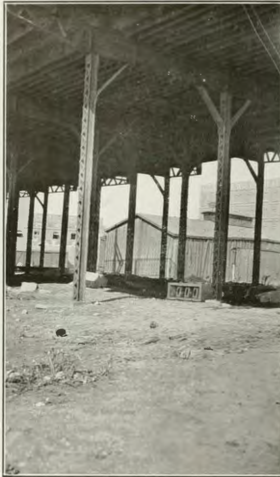
FIG. 49. WEST APPROACH TO FIRST STREET VIADUCT View of understructure, showing insufficient support.
