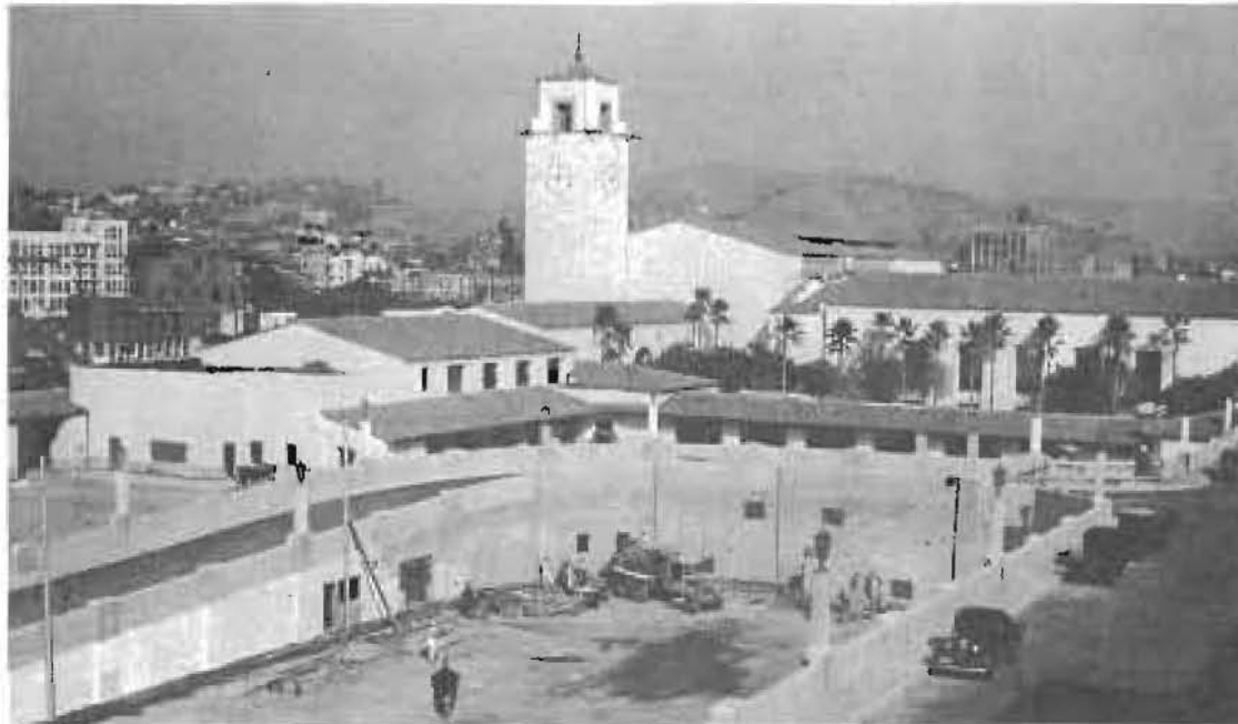
THE WIRES were up, but the track had yet to be laid in the Pacific Electric coach yard, as crews finish laying concrete (above). Santa Fe Railway
