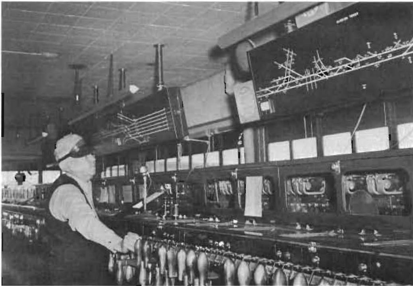
AT MISSION TOWER, 94 working levers control the following: 12 derrails, 28 turnout switches, six double slip switches, two turnout switches with movable point frogs, and 16 crossovers. Ninety-six more levers control 96 signals, and five levers control nine electric locks on switches that are not used frequently enough to warrant the expense of interlocking and handling from the tower. Seen here in 1947 is Santa Fe Towerman, E.L. Kelly, whose job also includes coordinating movements with the station's Terminal Tower. Stan Kistler
