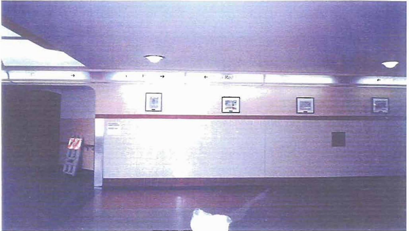
NON-HISTORIC TILE WAINSCOT IN TUNNEL; BORDER AT TOP IS PAINTED ON
