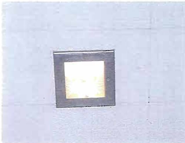
SQUARE CEILING LIGHTS FROM TRAIN CONCOURSE TO BE REMOVED AND REINSTALLED IN NEW RESTROOMS
