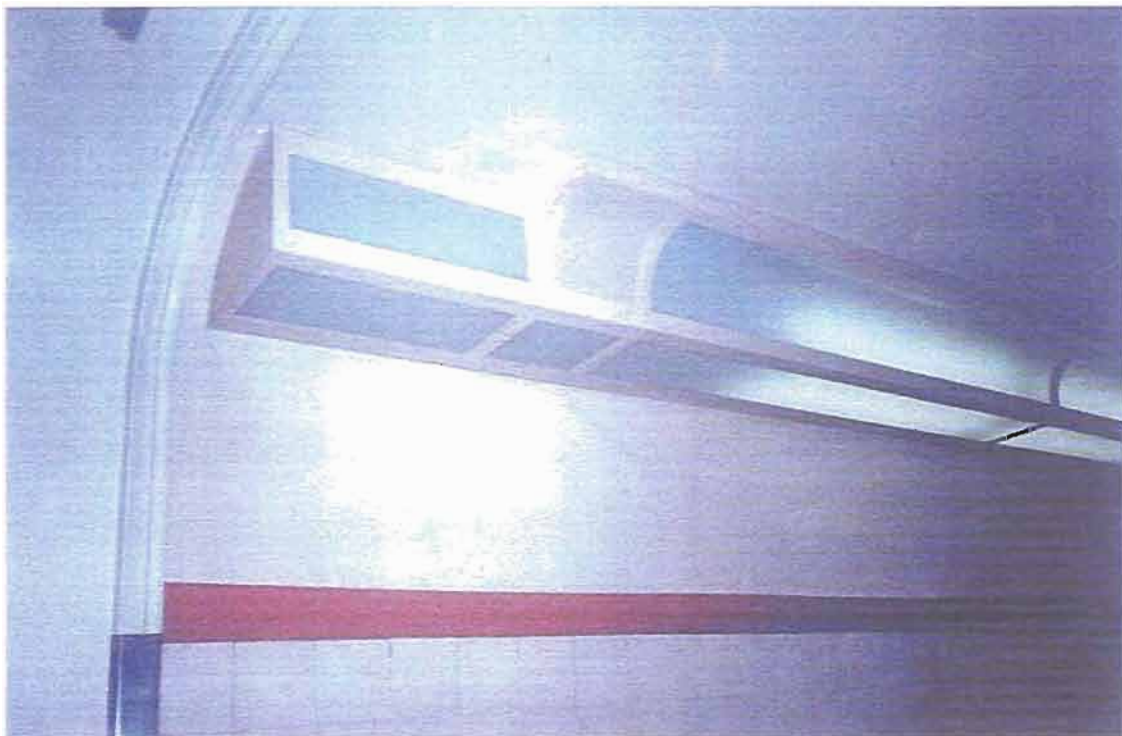
WEST END OF (NON-HISTORIC) COVE LIGHT FIXTURE AND COVERED CEILING PROFILE OF TUNNEL
