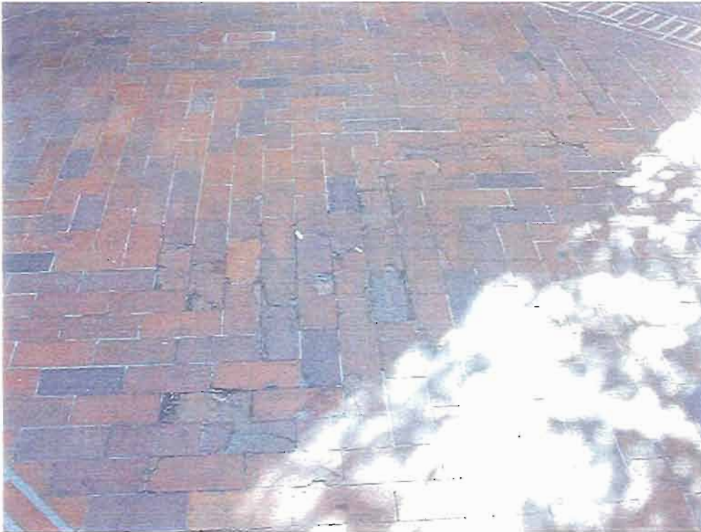
EXAMPLE OF DAMAGED PAVING TO BE PATCHED WITH REPLACEMENT BRICK WHERE NECESSARY
