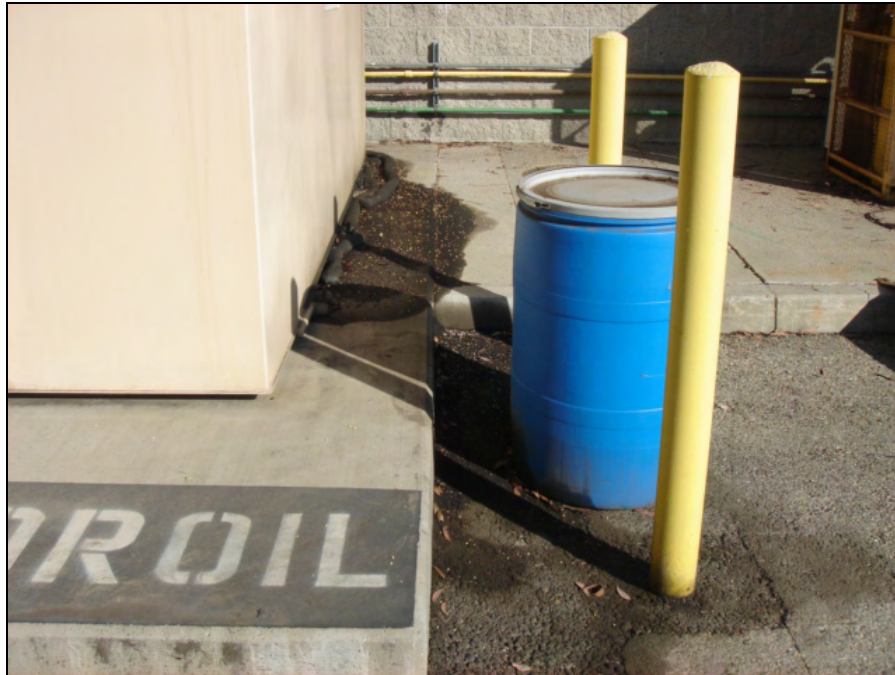
View of released oil from faulty pump system at top of tanks in Area 2
