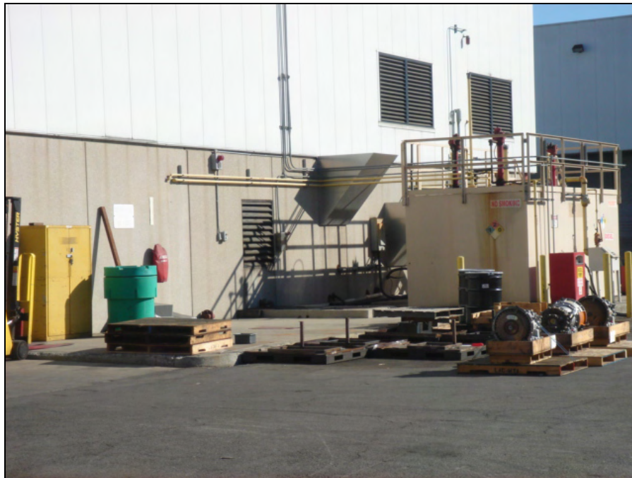
View of above ground diesel tank with pump in Area 2
