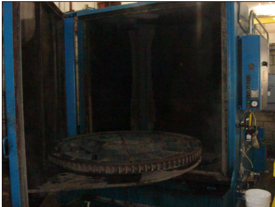
View of large parts, enclosed steam cleaning unit in Building 1
