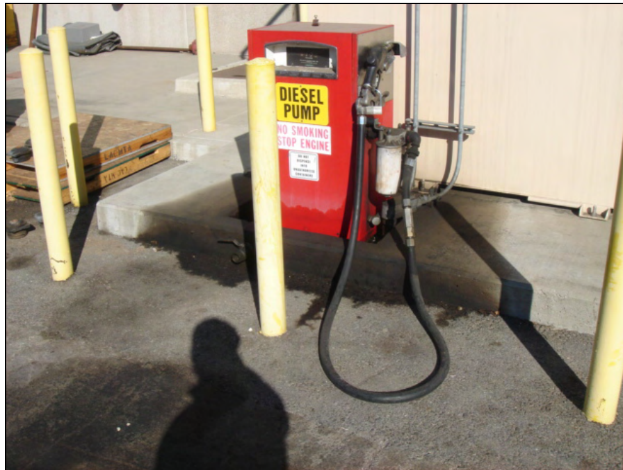
View of diesel dispenser in Area 2
