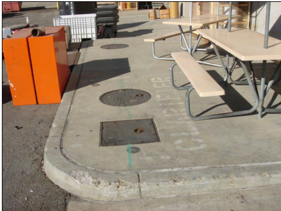
View of Clarifier in Area 2 South of Building 1
