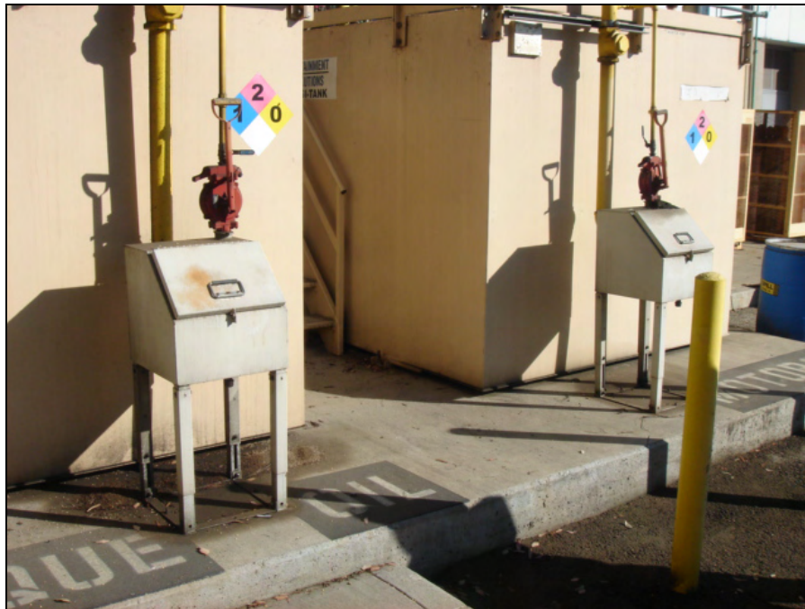
View of two 4,000 gallon, above ground, oil holding tanks in Area 2
