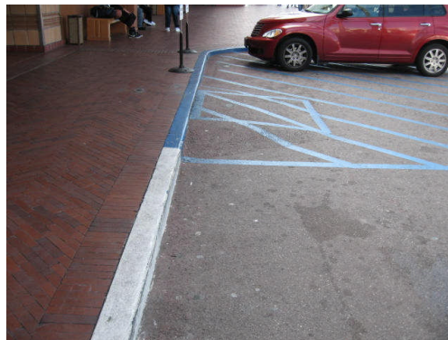
The ramp must be made of concrete, cannot be part of the loading zone, and ramp is not long enough, and there is no space for parallel parking
