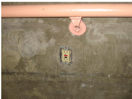
No cover on electrical outlet on ramp serving Tracks 11 and 12.
