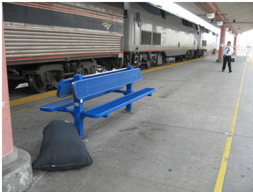
Bench on platform that does not meet the ADAAG requirements.
