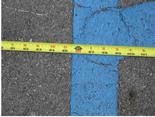
Parking stall is 8' wide; 9' is required
