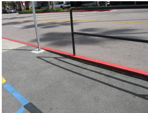
The ramp to the parking spaces does not meet the ADAAG requirements for a stable surface.
