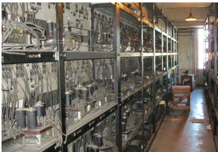
Switch equipment on second floor of Amtrak Switch Building.
