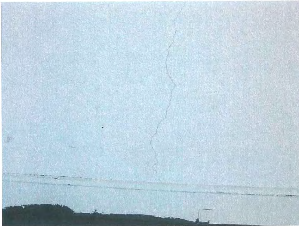
Photo #3 – Typical crack in stucco at inside wall above counterflashing.
