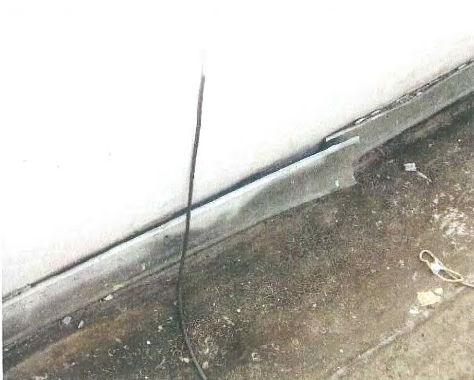
Photo #6 – Loose counterflashing at South clock tower well.
