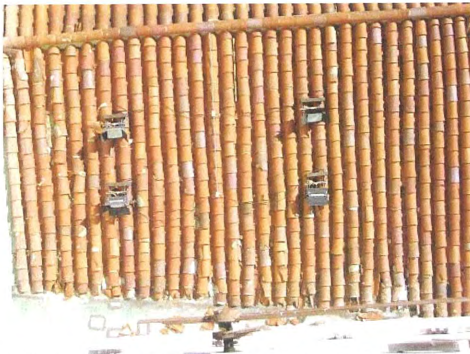
Photo #4 – Typical broken tile at base of East side of clock tower.
