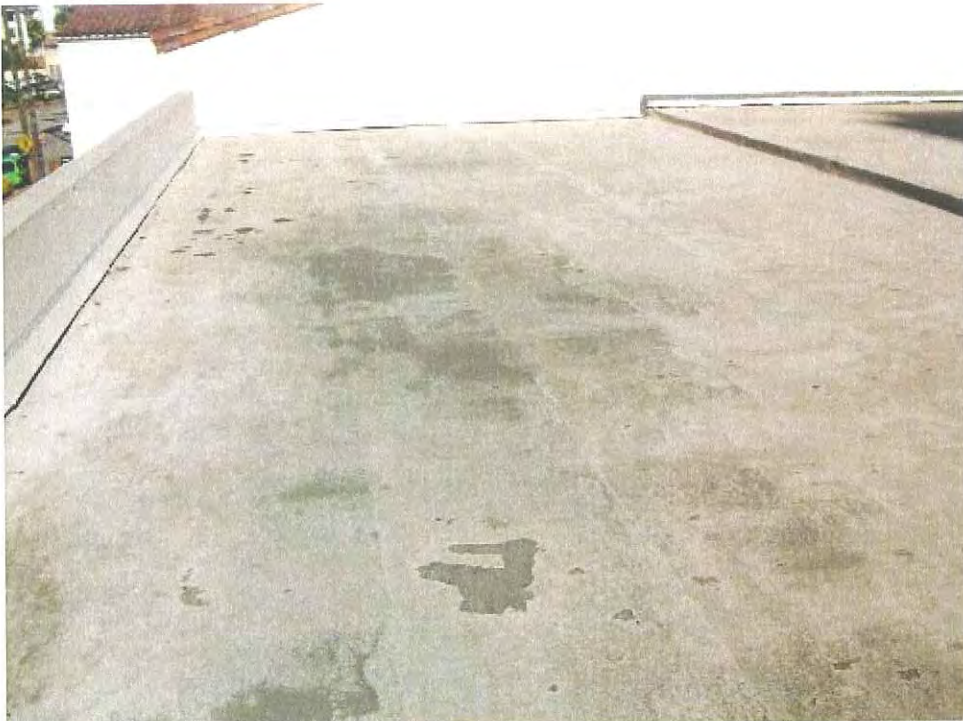
Photo #7 - General overview of South built-up roof leak area.
