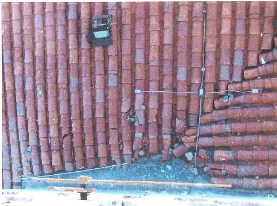
Photo #2 – Typical broken tile at base of North side of clock tower.
