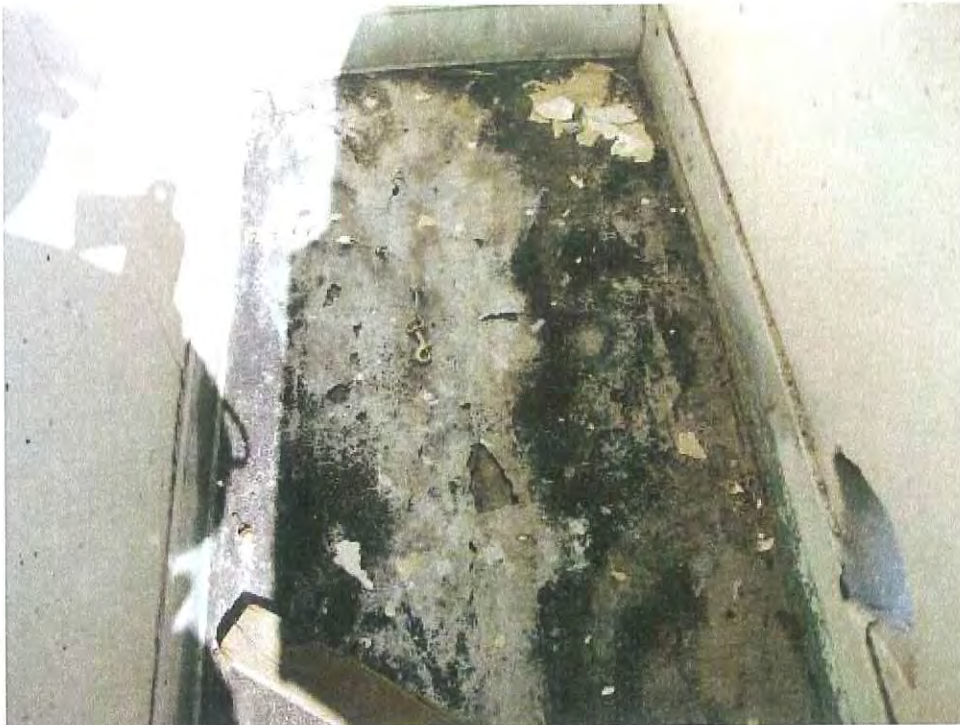
Photo #5 – Deteriorated roofing at East clock tower well.
