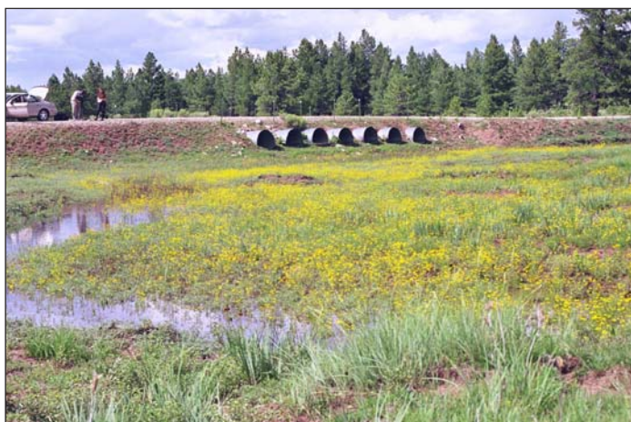
Install culverts with the invert elevation at a higher elevation than the meadow elevation in order to promote seepage and infiltration
