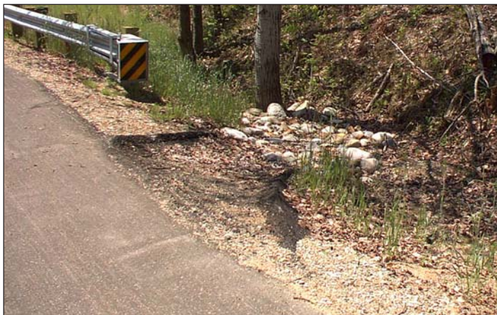
Lead out ditch with energy dissipater (Michigan)
