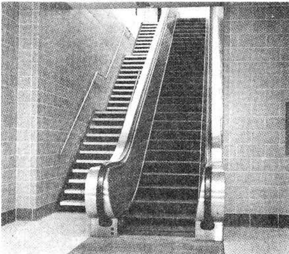
Escalator at passageway entrance at ground level in C&NW station MTD-5
