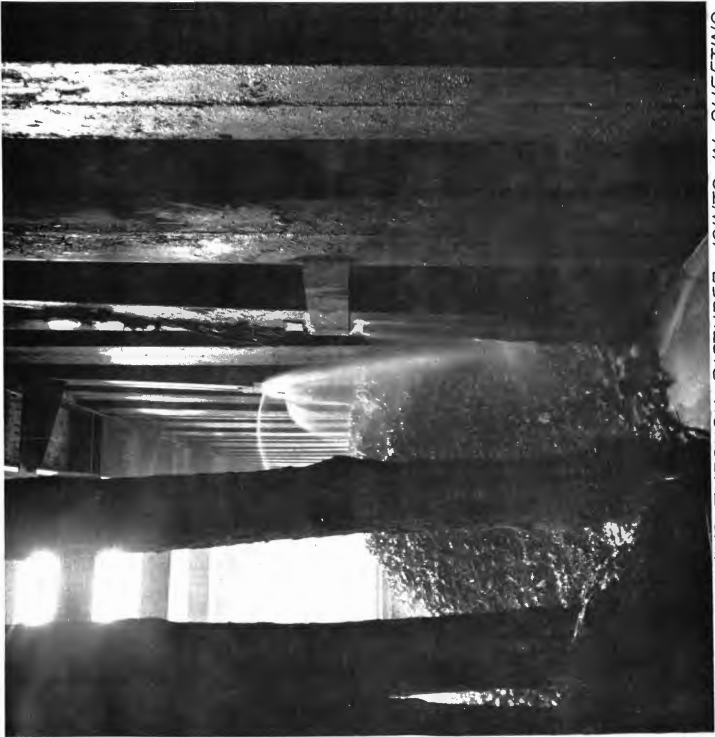
FIGURE 4.3 WATER FLOWING THROUGH RAPTURED JOINTS IN SHEETING TEST SECTION B (COMPLIMENTS OF MBTA)
