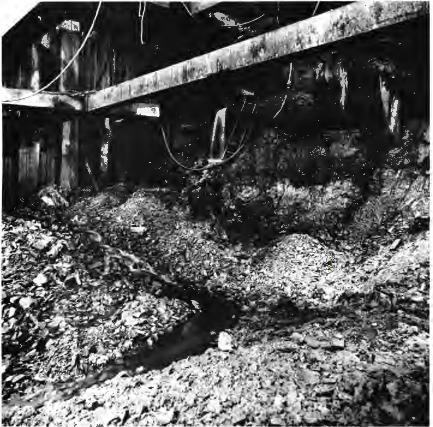
WATER FLOWING INTO EXCAVATION (Looking south from station 76+33, 12/17/68)
