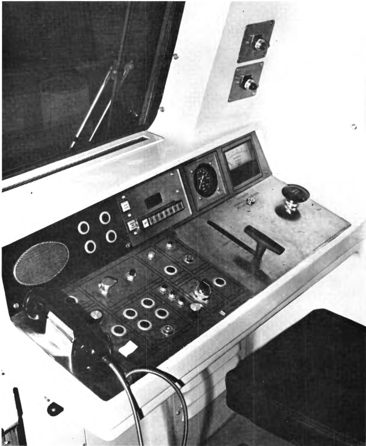
Figure 4-13. Master Controller Panel
