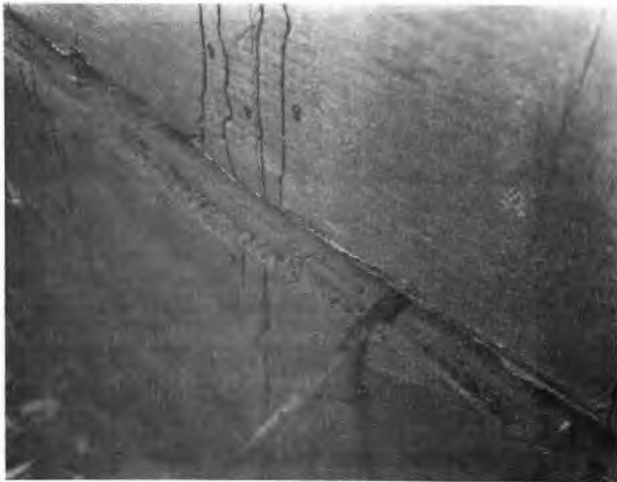
FIGURE 3.12 TOP VIEW OF ADHESION FAILURE DEVELOPED BETWEEN THE MORTAR LAYER AND THE CONCRETE SLAB COVERING THE MOVABLE BLOCK IN TEST NO. 15
