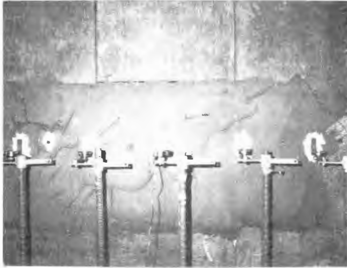
FIGURE 3.1 PRE-TEST SURFACE CRACKS IN TEST NO. 1
