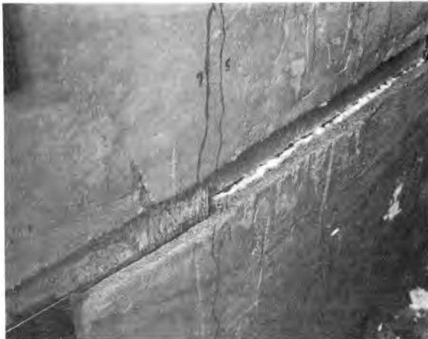
FIGURE 3.9 STEEL PLATES PROVIDING RESTRAINT TO ADHESION FAILURE PROPAGATION
