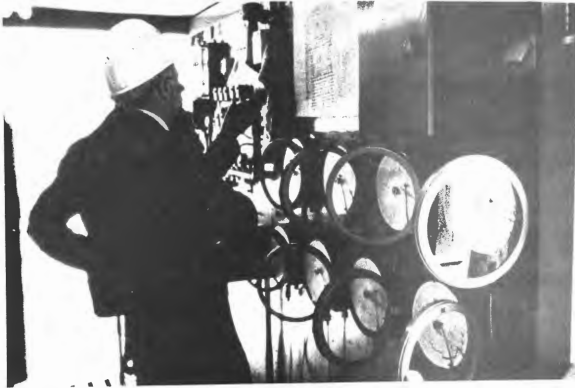
Figure 52. Recording gauges and pump controls in grouting trailer.
