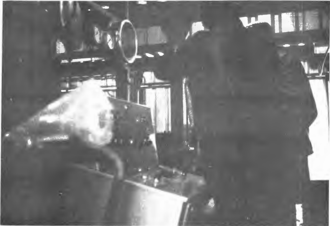
Figure 50. Electronic console for grout pump automation.
