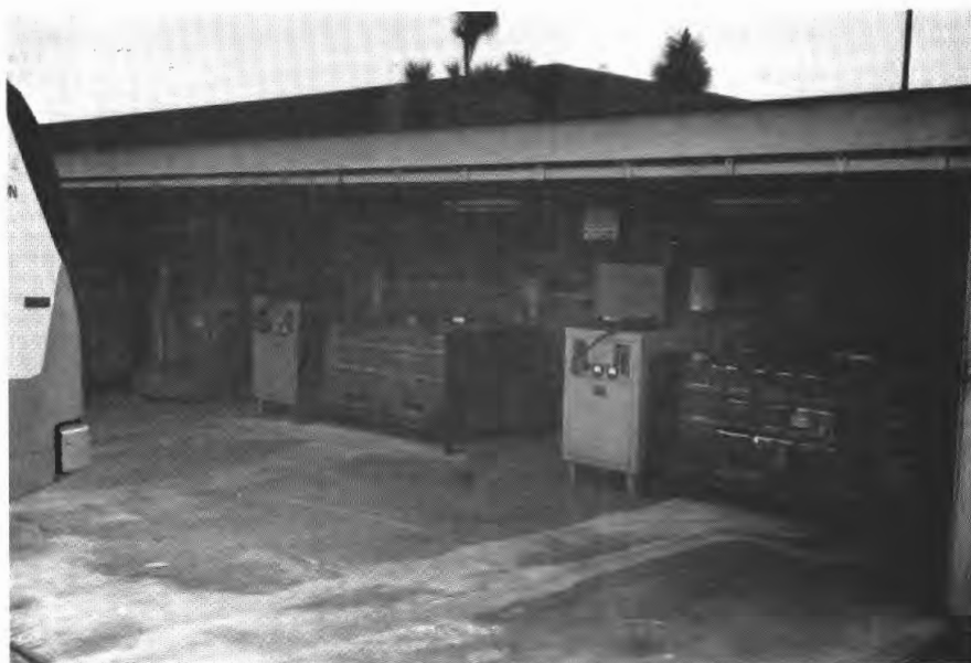
Figure 3-2. Battery Maintenance Facilities, Long Beach
