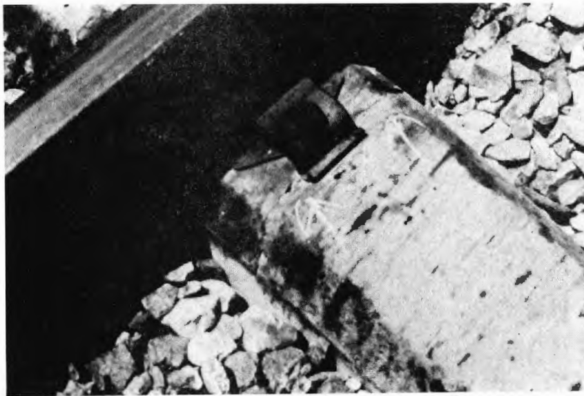
Photo #3 - Rail Seat Crack - also showing bolt failures, tie pad deterioration and fines from ballast degradation. Tie removed from track during ballast replacement operation (2)
