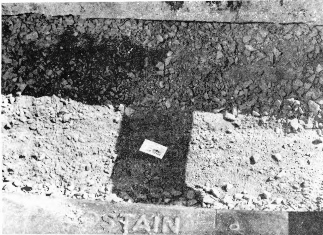
Photo #23.- Migration of Subgrade Fines Into Ballast, Concrete-Tie Subsection E (3)
