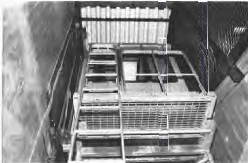
Lower end of inclined elevator car, showing exterior platform and ladder used for maintenance and emergency evacuation.
