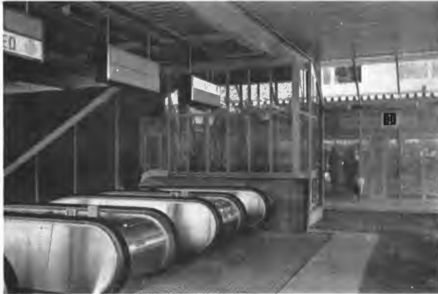
Fare hall landings of escalators and inclined elevator enclosed with glass and metal mesh.
