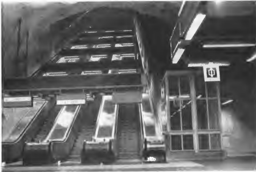
Lower landing of escalators and inclined elevator in cross-passage leading to train room.
