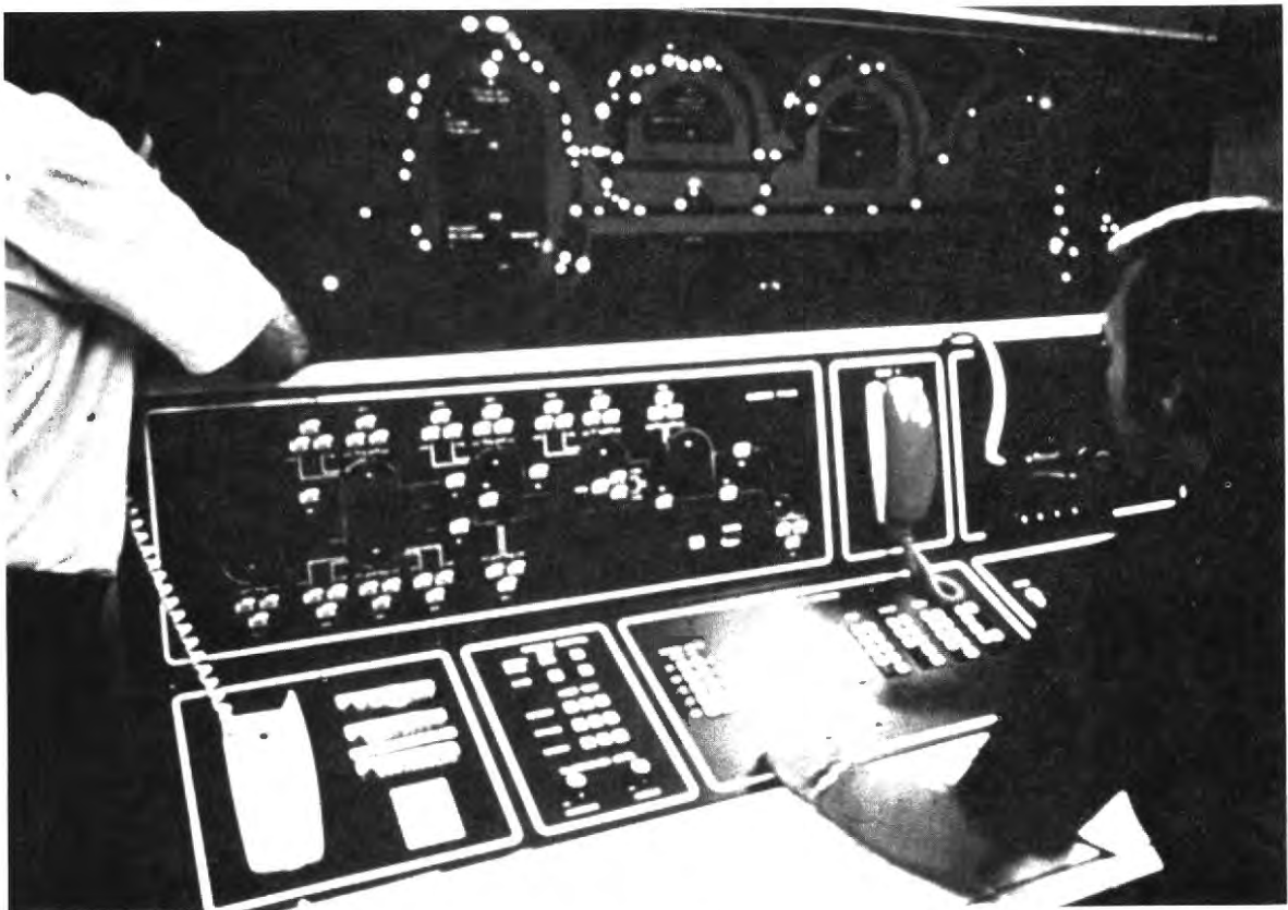
FIGURE 7 CENTRAL CONTROL SYSTEM USED TO MAINTAIN SAFE VEHICLE OPERATING CONDITIONS FOR THE AIRTRANS AGT SYSTEM AT THE DALLAS-FT. WORTH AIRPORT IN TEXAS
