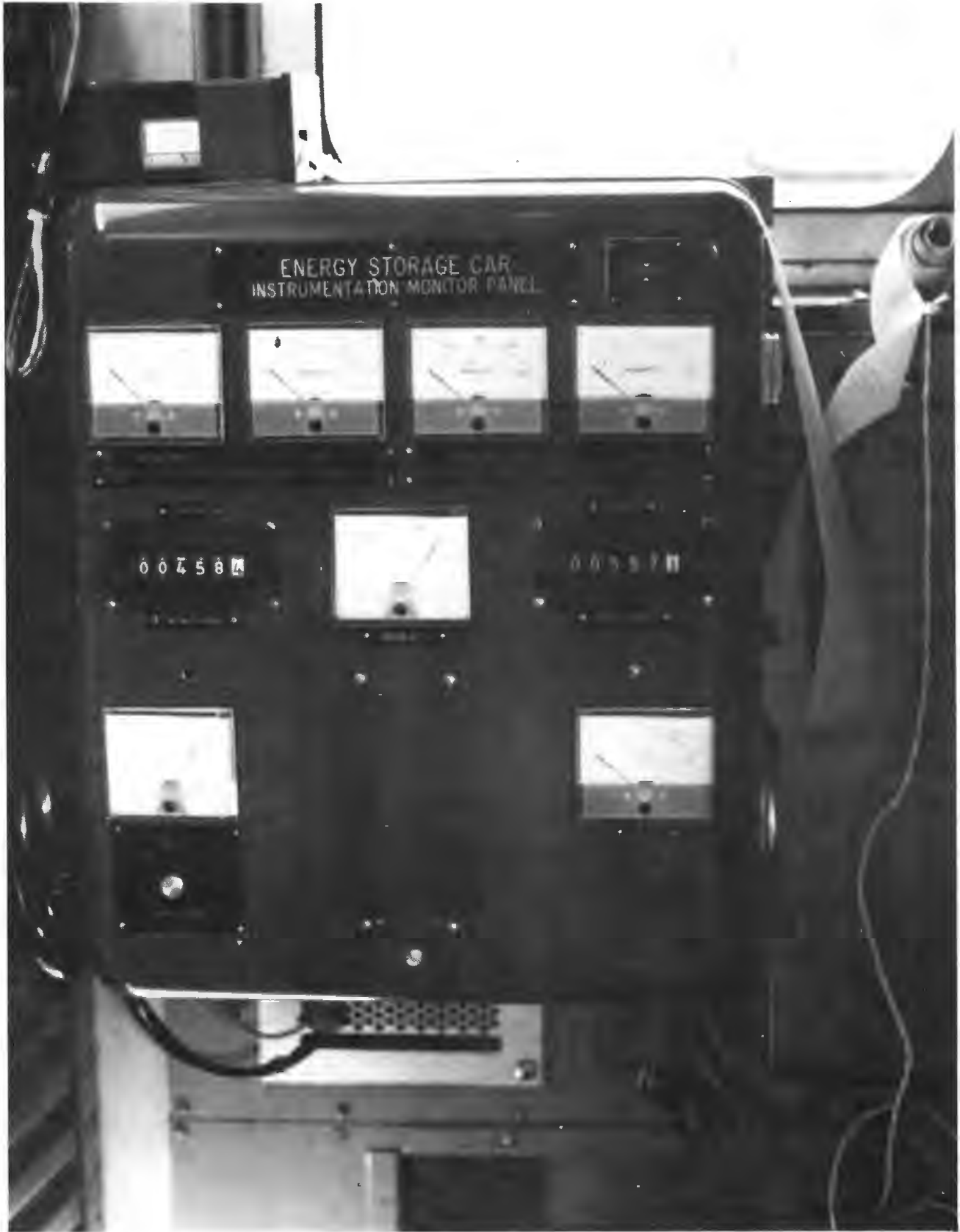
Figure B-3. Energy Metering and Monitoring Panel
