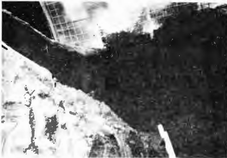
Figure 4.8 Close-up of Crown and Side Wall during Tunneling for the Bochum Metro
