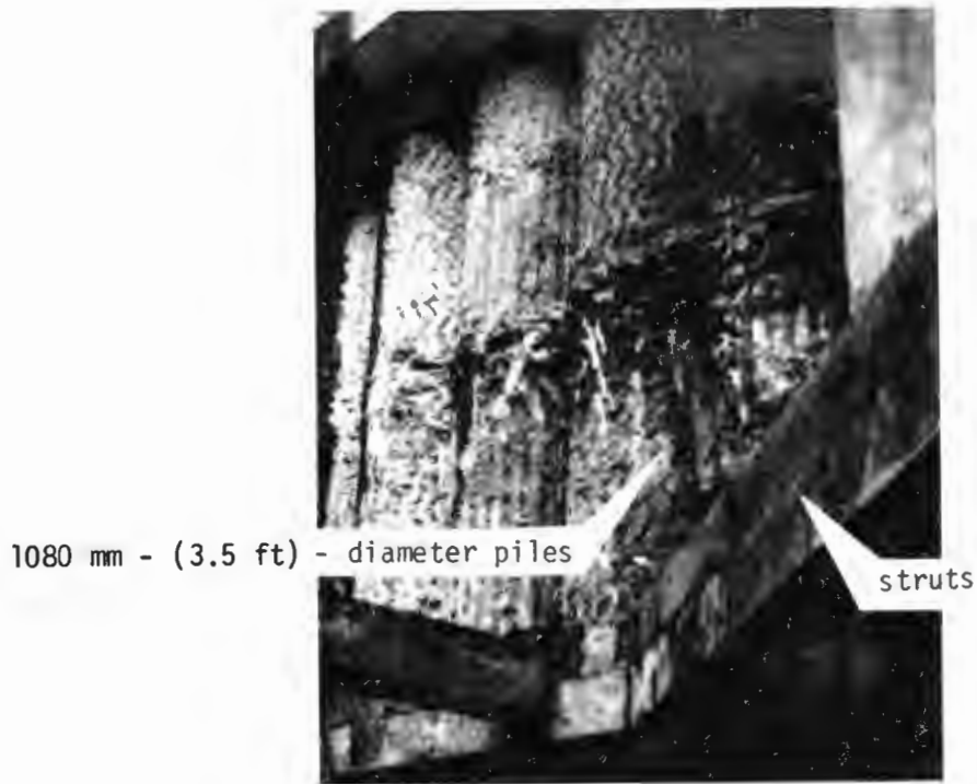
Figure 3.16 Secant Pile Wall for Monument Station on the Tyne and Wear Metro.
