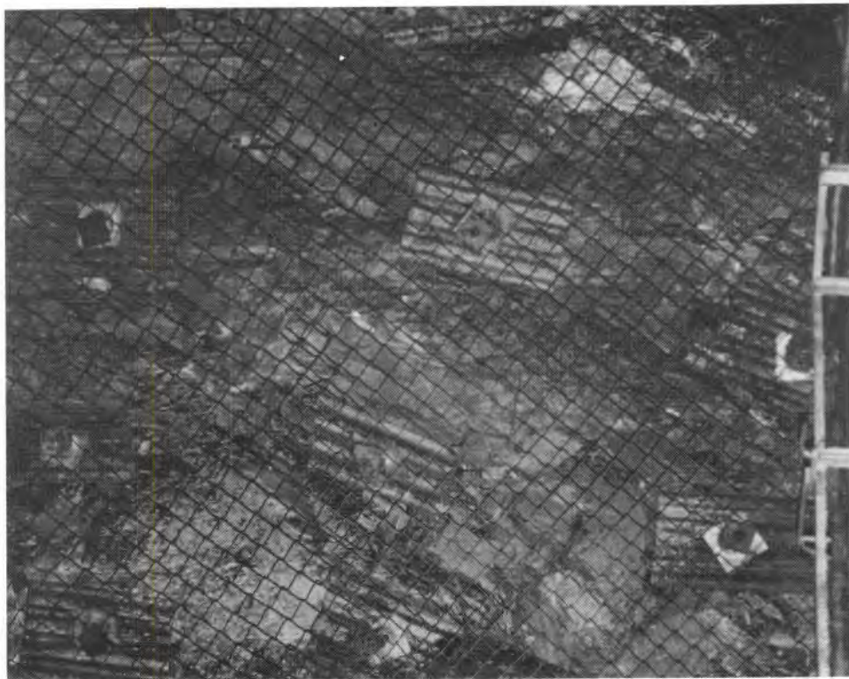
PLATE AIV-20. Wire mesh and rock bolts with flexible bearing plates
