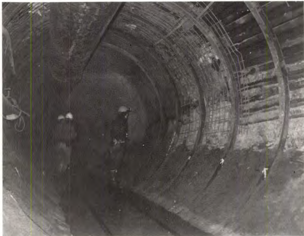
PLATE AIV-9. Shear zone ground support of continuous lagging and circular steel sets spaced on one meter centers, Tees station 4303 to 4310
