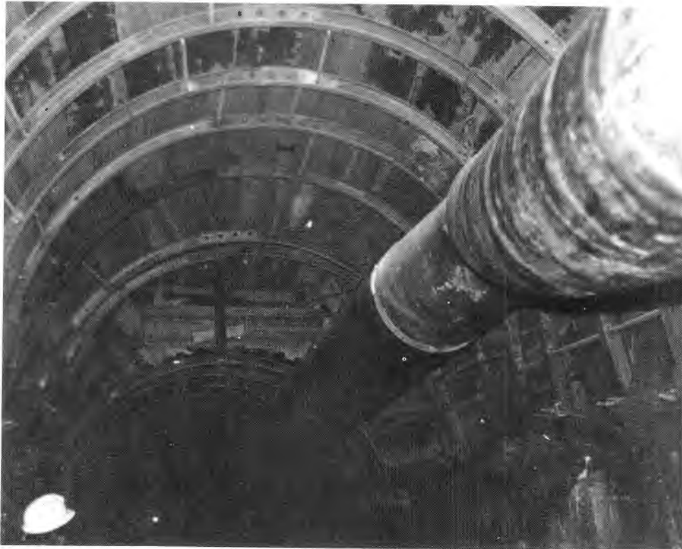
PLATE 3-4. Overbreak in very blocky mudstone
