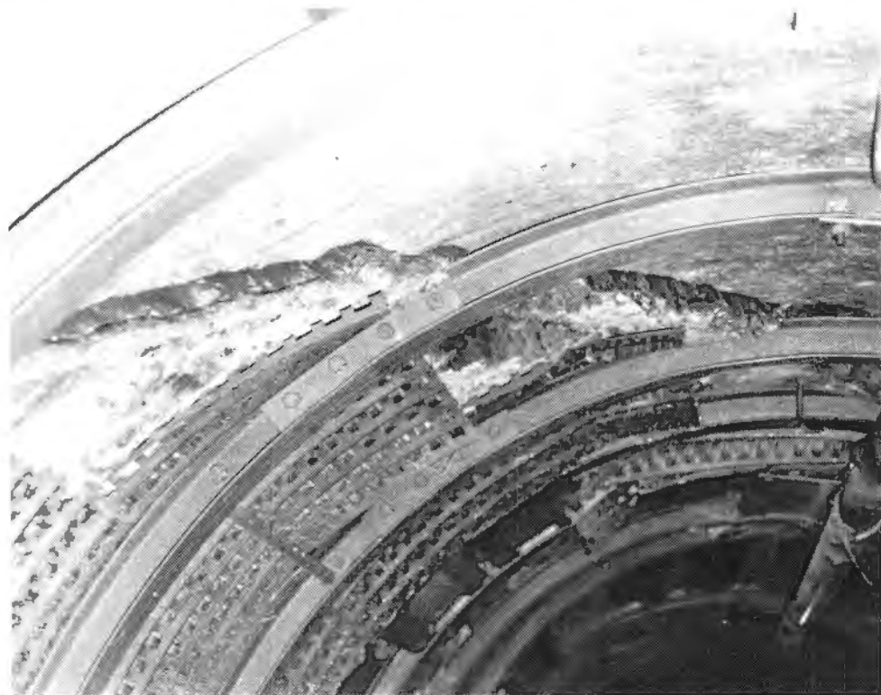
PLATE AIV-7. Transition between fault gouge showing minor squeeze and massive limestone, Tees station 1295
