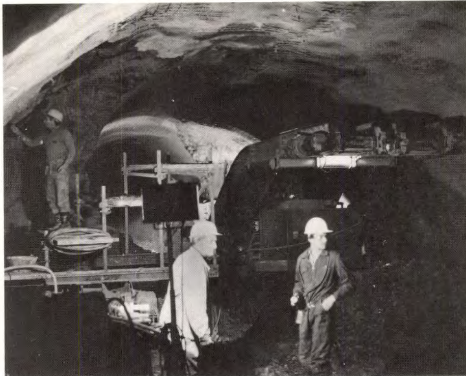
PLATE AIV-17. Construction of top heading with excavation by Westfalia roadheader; note pilot tunnel
