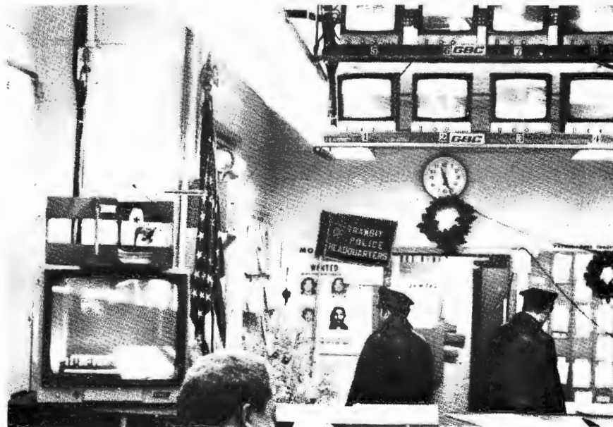
FIGURE 2.1.8. THE CLOSED-CIRCUIT TELEVISION MONITORING FACILITY FEATURES MONITORS, A TIME LAPSE VIDEO RECORDER, AND A PUBLIC ADDRESS SYSTEM
