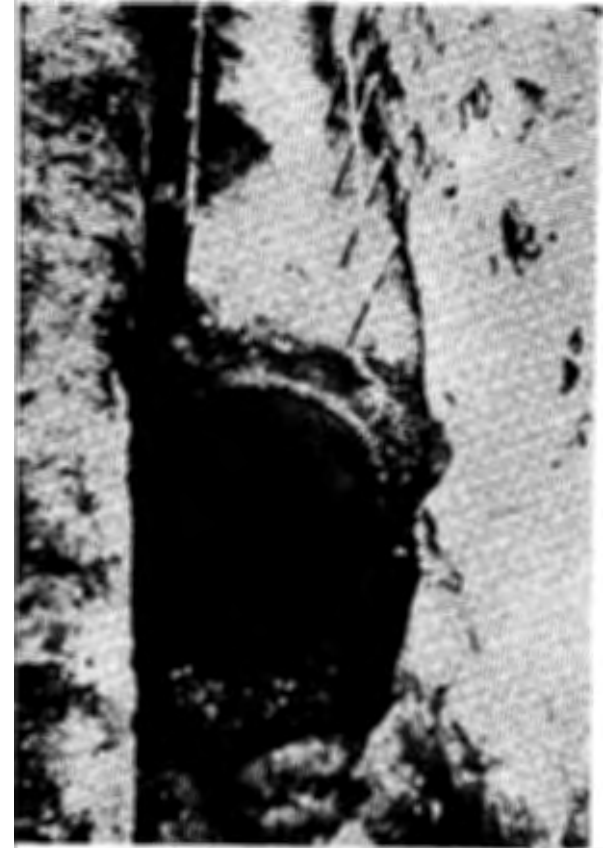
FIGURE 13 FIELD PHOTO OF A HALF-ROUND JOINT FORMED BY USING A STOP END PIPE
