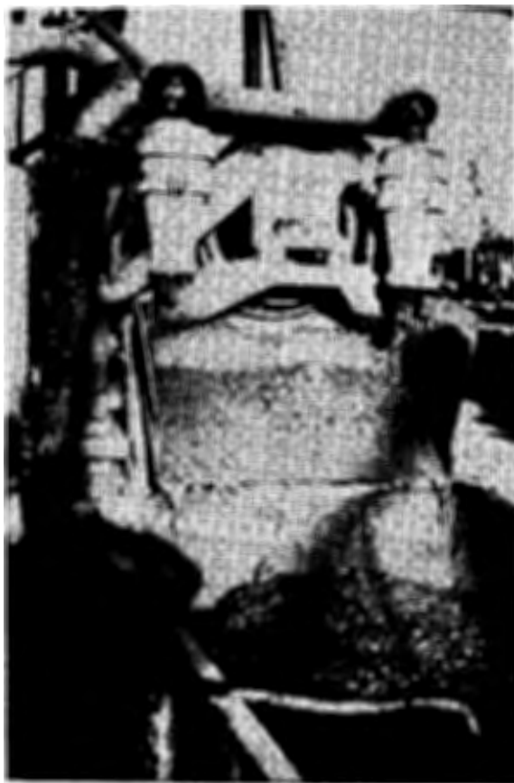
FIGURE 15 FIELD PHOTO OF RESIDUE FROM DESANDING UNIT
