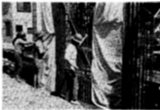
Fig. 5 Vinylon-sheet and steel-plate joint. (a) General joint detail and splicing of horizontal reinforcement. Note that the interlocking pipe is not shown. Concrete is poured against the vertical steel plate. (b) Detail showing the attachment of vinylon sheet to the steel plate. (c) The reinforcement cage is lowered into the trench; vinylon sheets are extended 3 to 4 ft to prevent concrete from leaking into the next panel.
